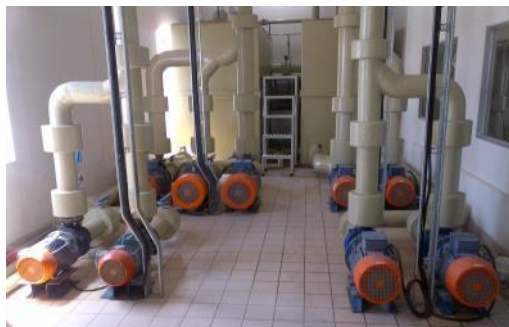
Figure 5. Upgraded AC1 recirculation pumps.
