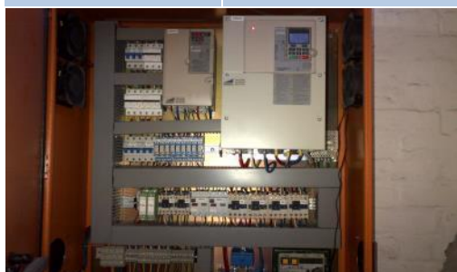
Figure 4. Cooling Fan and Pump VSD Controller in Dairy PET Department.
